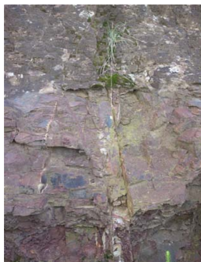
Figure 3.13: Through going joint in the type section at Bald Hill, just north of Stanwell Park.
